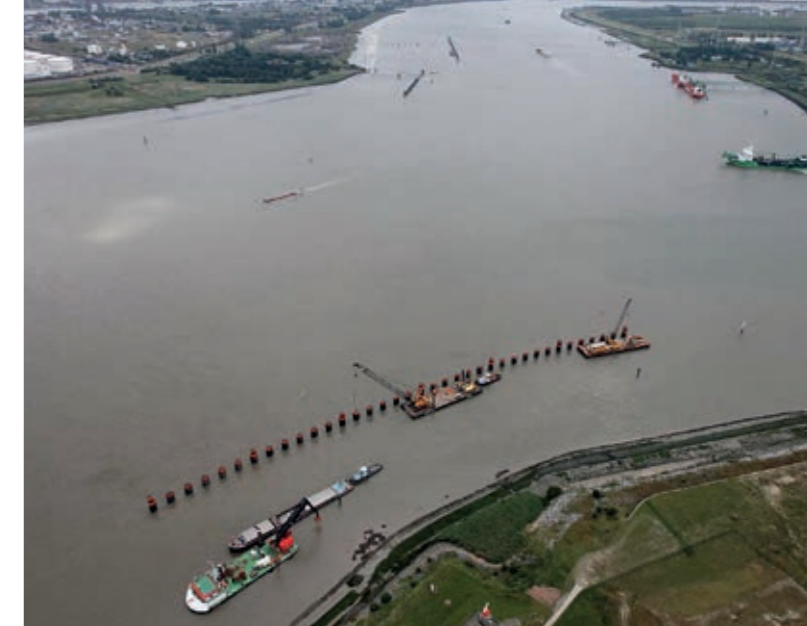
Construction of a current-deflecting wall with the ALBATROS in the Port of Antwerp, Belgium.
