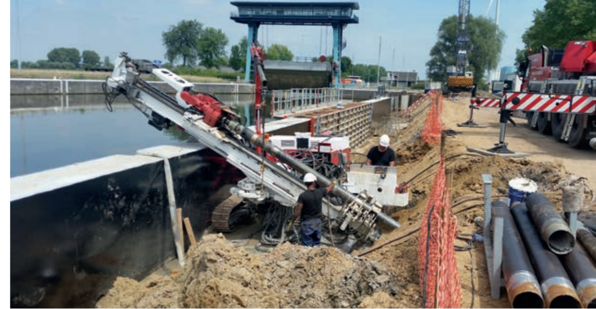
Installation of ground anchors to stabilise the new quay wall in Sint-Baafs-Vijve, Belgium.
