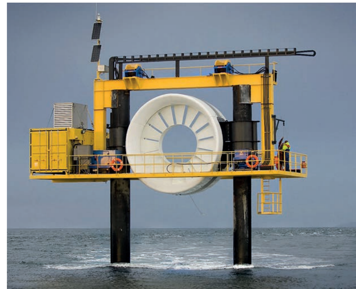
Installation of the UK's first grid-connected tidal turbine using the Octopus, Orkney Islands.
