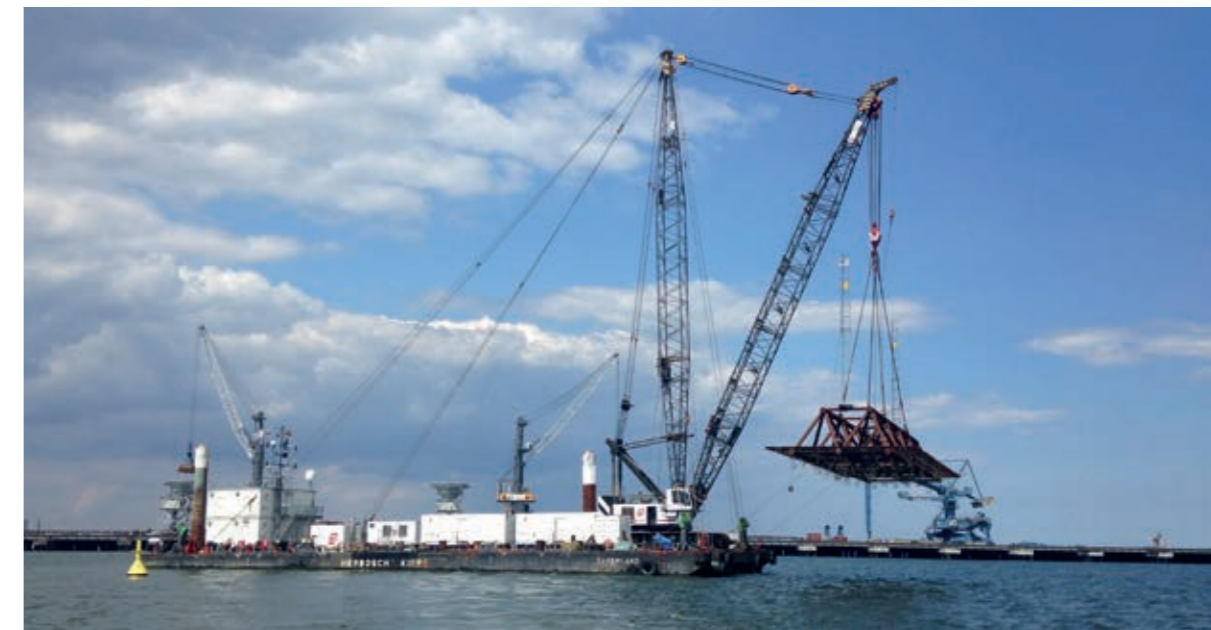
Fabrication and installation of asphalt mattresses weighing approx. 200t, for scour protection in Gdansk, Poland.
