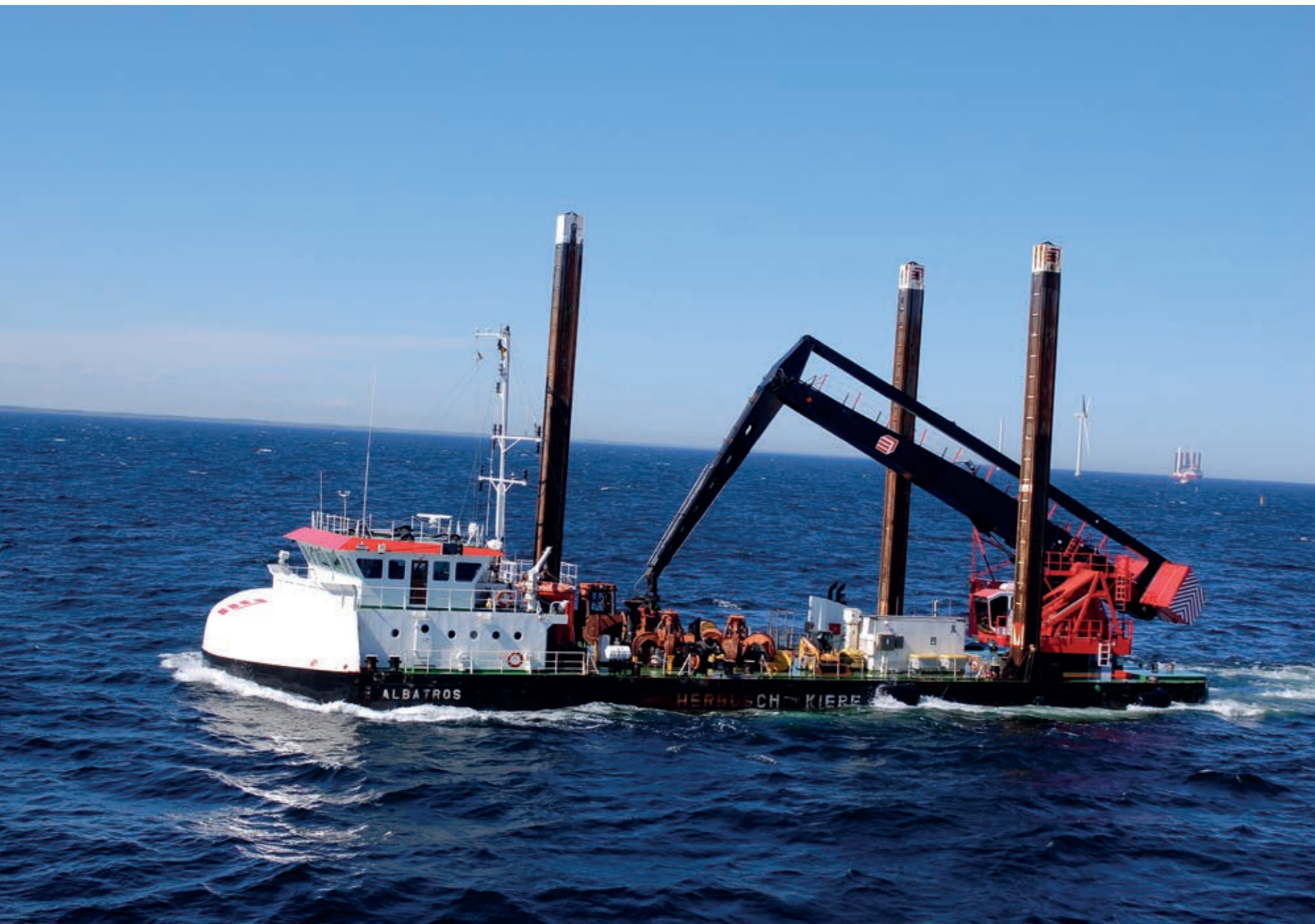
The ALBATROS working on the construction of wind farm foundations for the Kårehamn Offshore Wind Park, Sweden.
