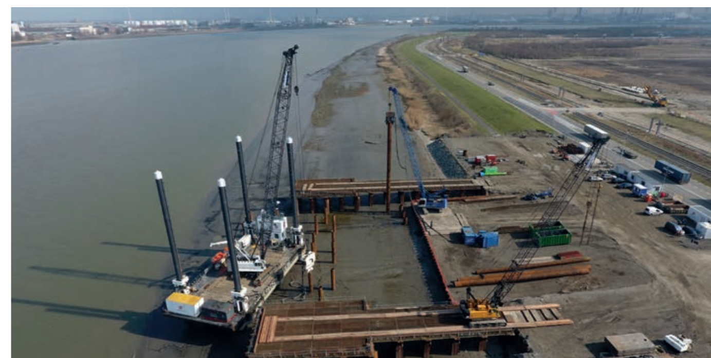
Piling works for the construction of two new pylons 192m high on the banks of the River Scheldt, Belgium.
