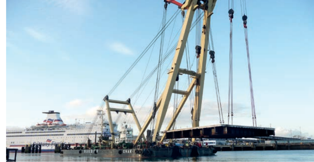
Demolition and removal of the Floating Dock Jetty in Portsmouth, UK. The deck of the jetty was cut into 18 sections, some weighing as much as 400t.
