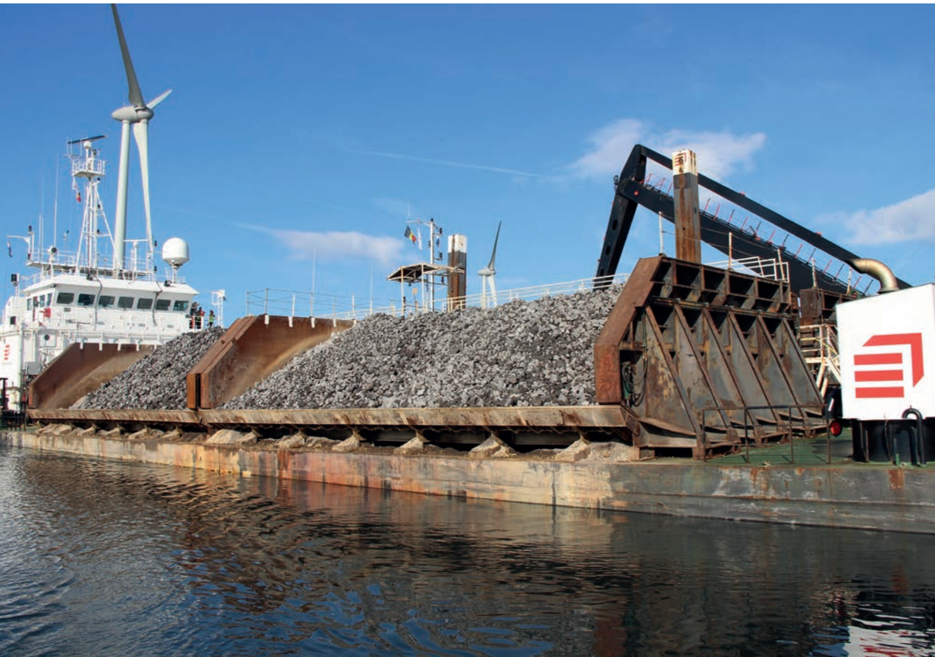
The ATLANTIS rock dumping for protection and stabilisation works on the Oosterschelde storm surge barrier in the Netherlands.
