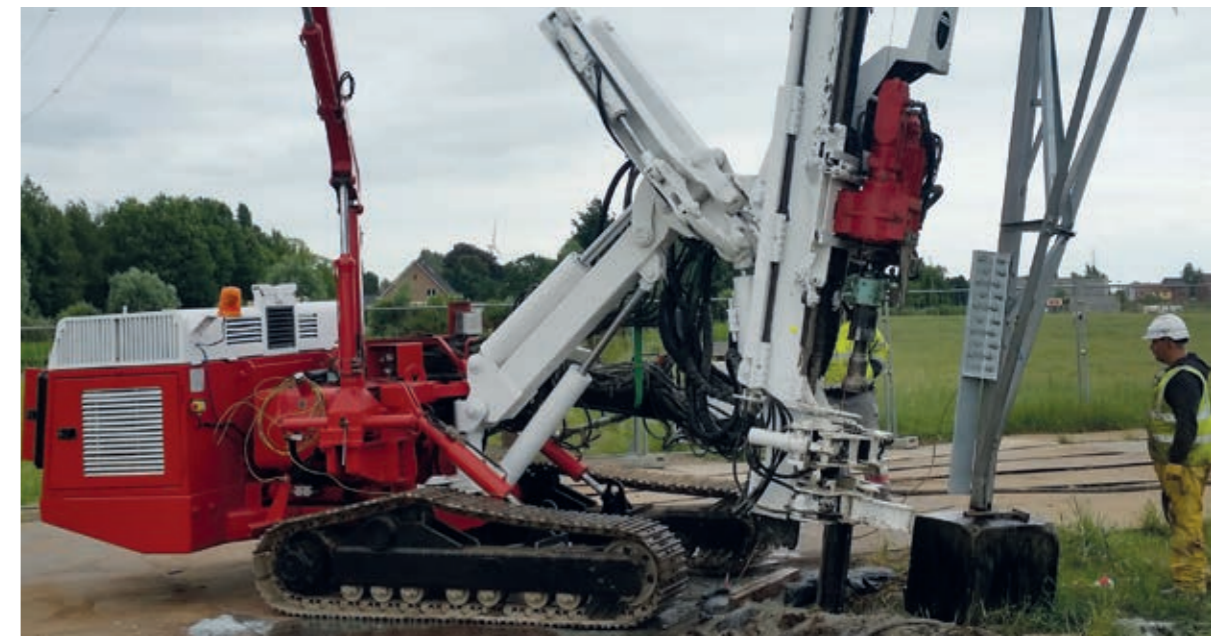
Installation of micropiles to reinforce the foundations of 26 of Elia's electricity pylons, Belgium.
