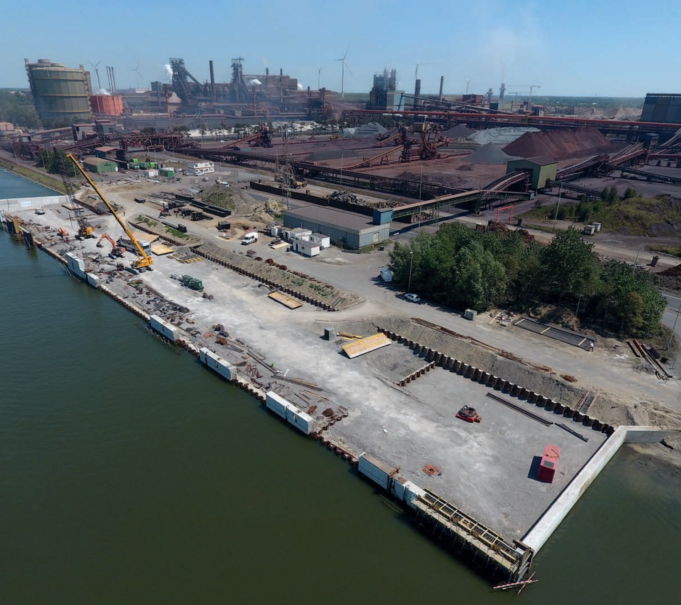
Construction of a 220m quay wall in the Port of Ghent, Belgium.
