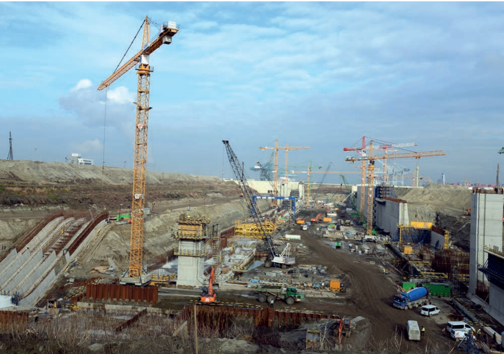
Construction of a lock (500m x 68m) in Waasland Port, Port of Antwerp, Belgium.
