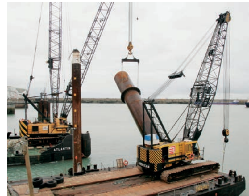
Extension of Pier E to accommodate the arrival of new, longer passenger ships in Dover, UK.
