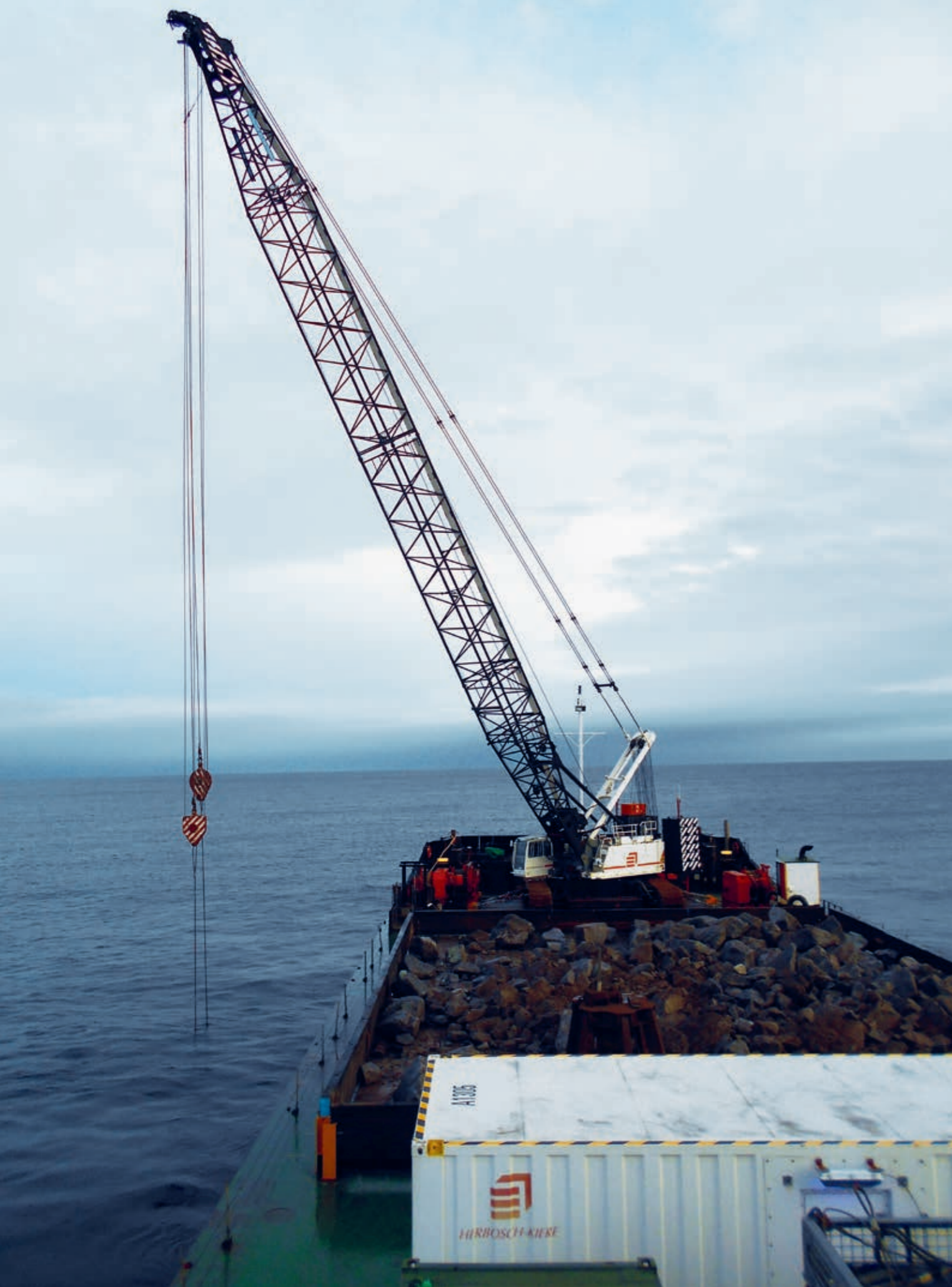
Rock placement by the ATLANTIS to protect subsea cables close to Noss Head, Scotland.
