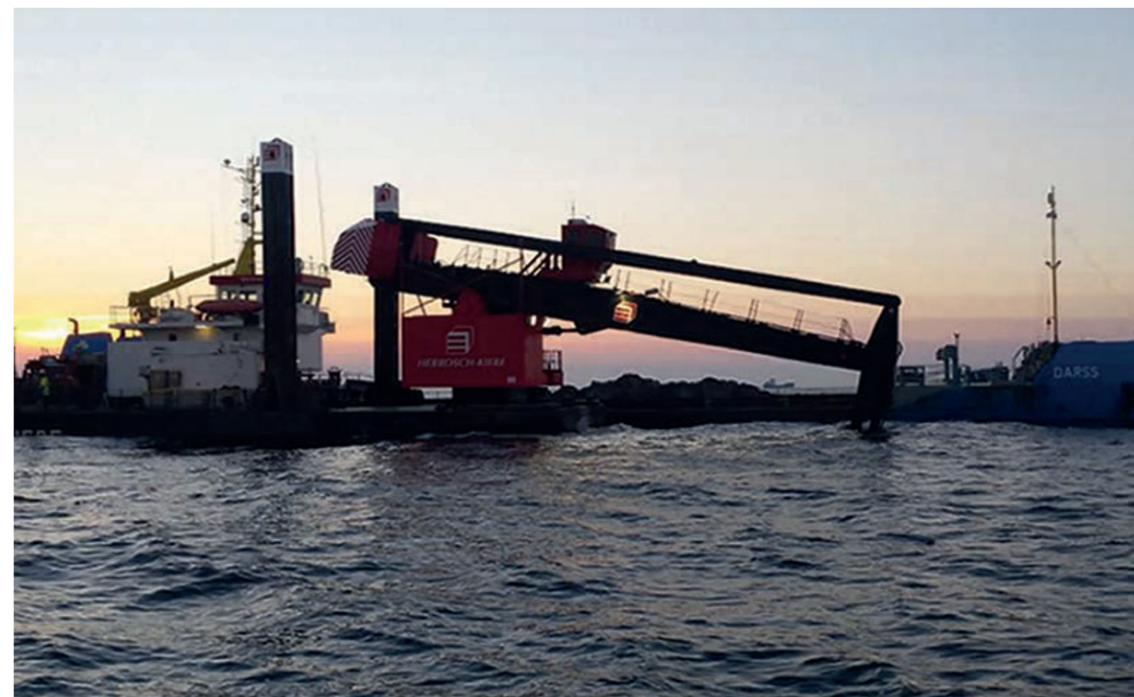
Dredging works for cable laying using the ALBATROS on the Westliche Adlergrund Windpark, Germany.
