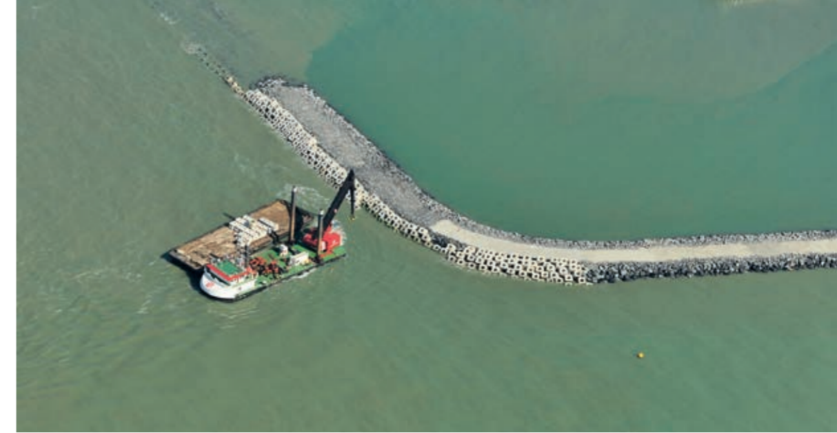
Construction of harbour breakwaters in Ostend, Belgium, with two of our vessels: the ALBATROS and the ATLANTIS.
