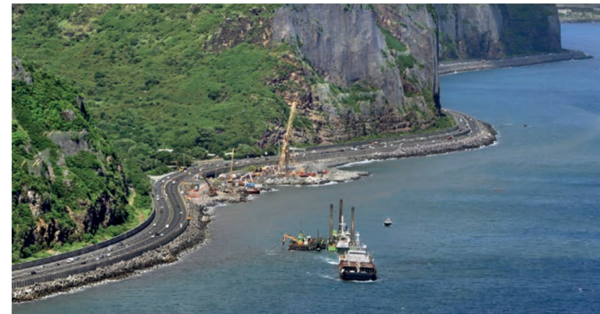
The ATLANTIS rock placing for the new coast road viaduct on Réunion Island in the Indian Ocean.
