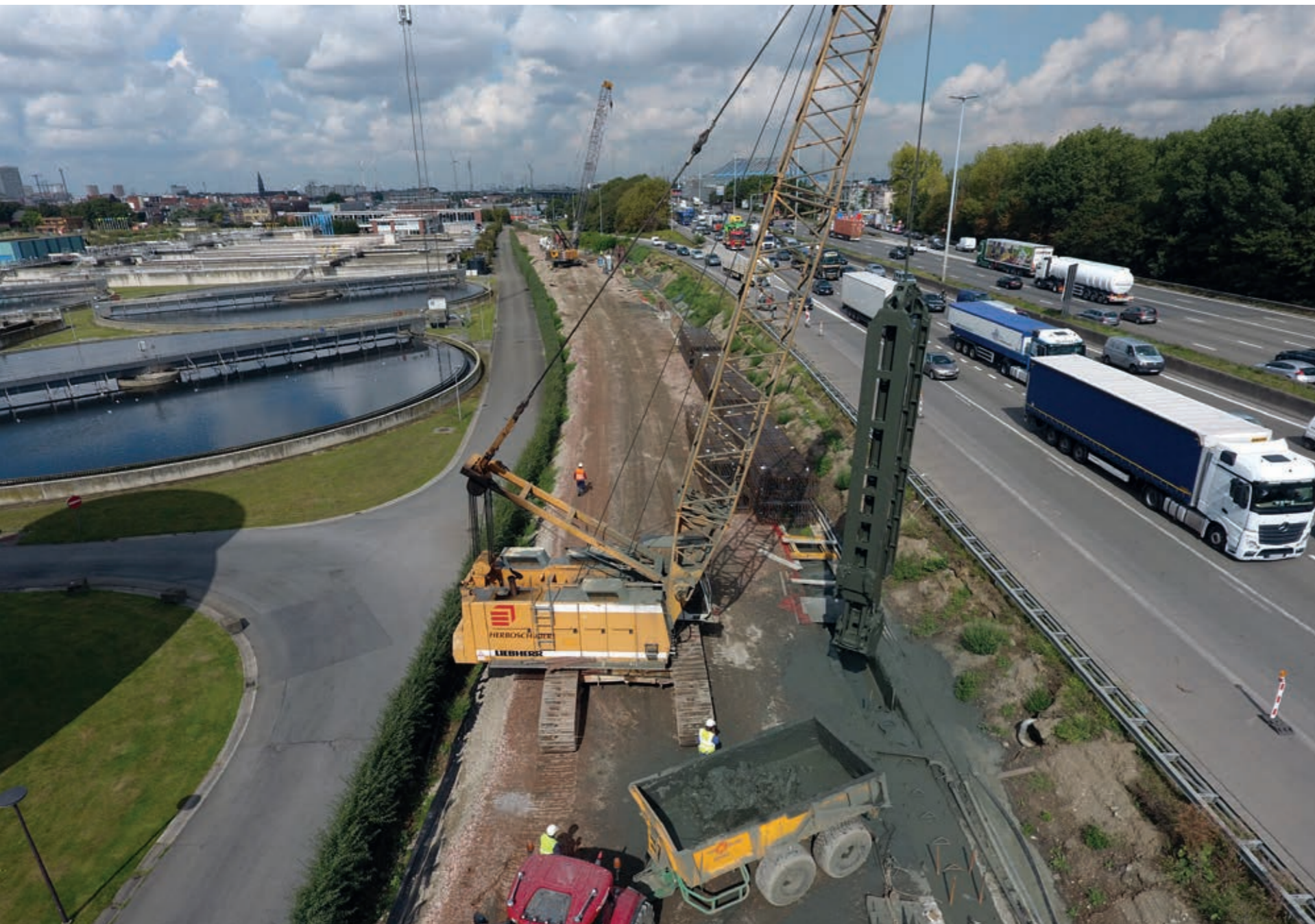
Construction of diaphragm walls up to 42m made of reinforced concrete for the Oosterweel Project.
