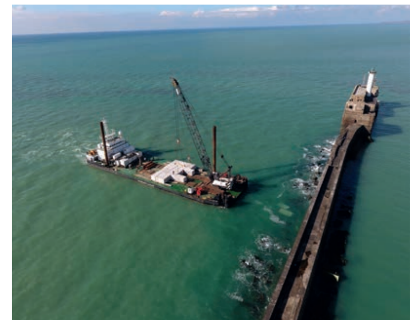
Placement of 500 concrete blocks of 50t and 33t by our multi-purpose vessel, the ATLANTIS, in Boulogne, France.
