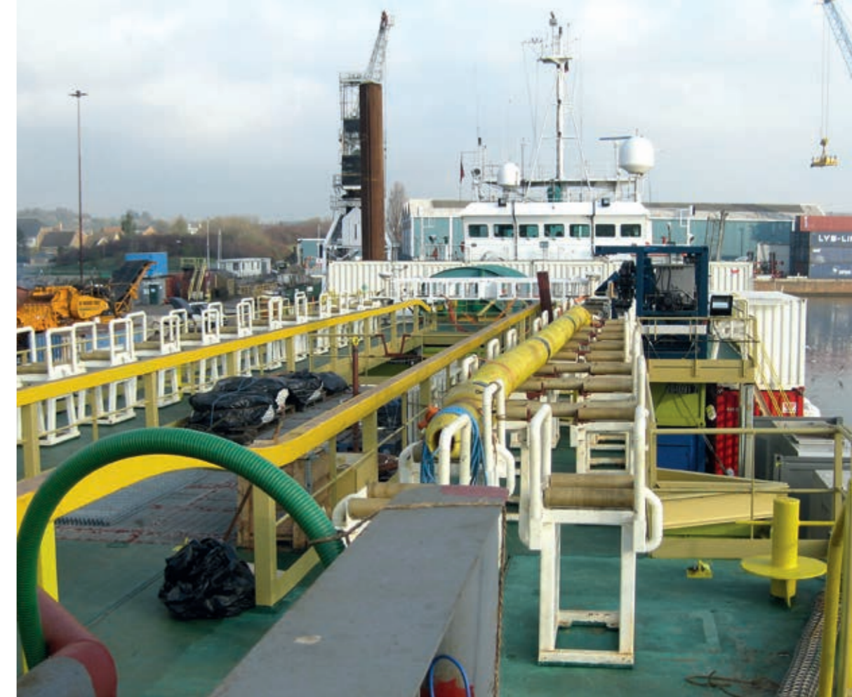
Installation of 33kv transmission cables by the ATLANTIS on the London Array wind farm, UK.
