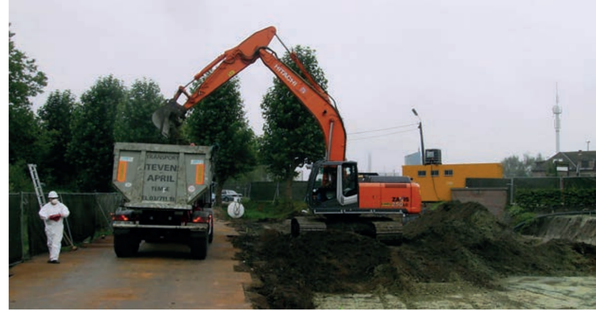
Excavation of 21.000m 3 of radioactive soil and sludge from a Umicore site, Belgium.
