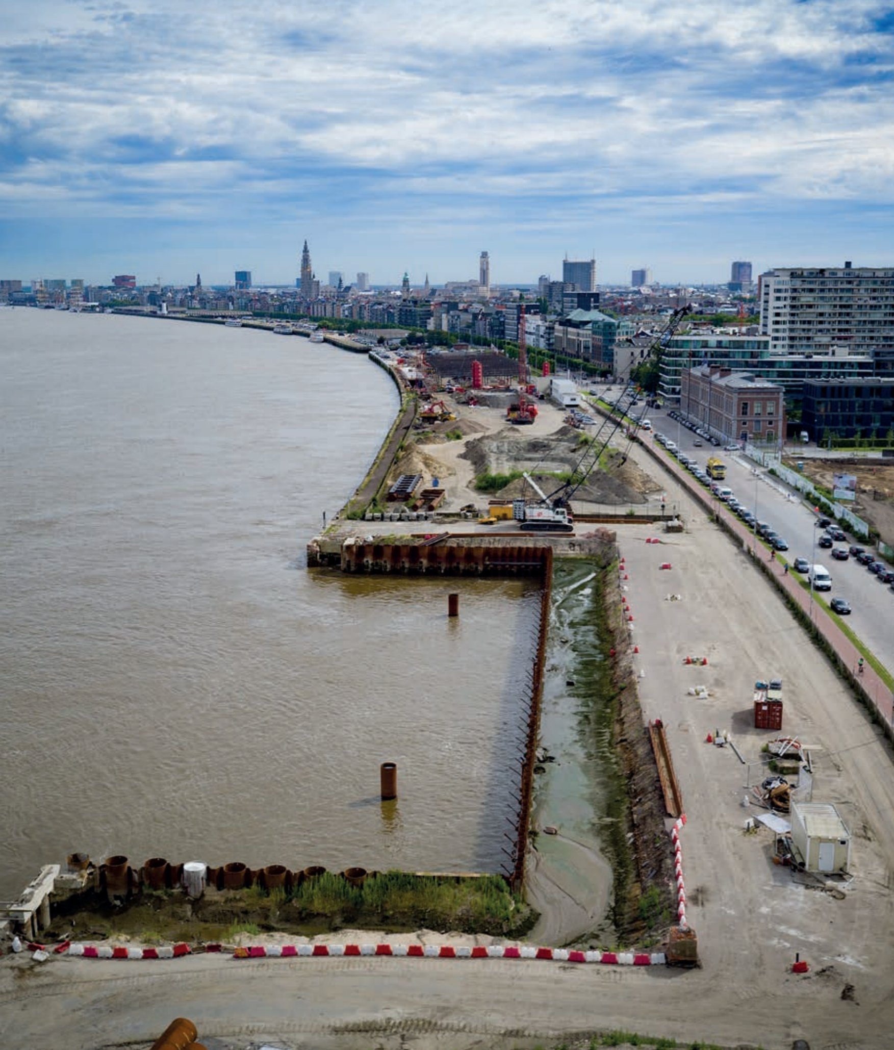
Reconstruction of a 700m quay wall in the City of Antwerp, Belgium.
